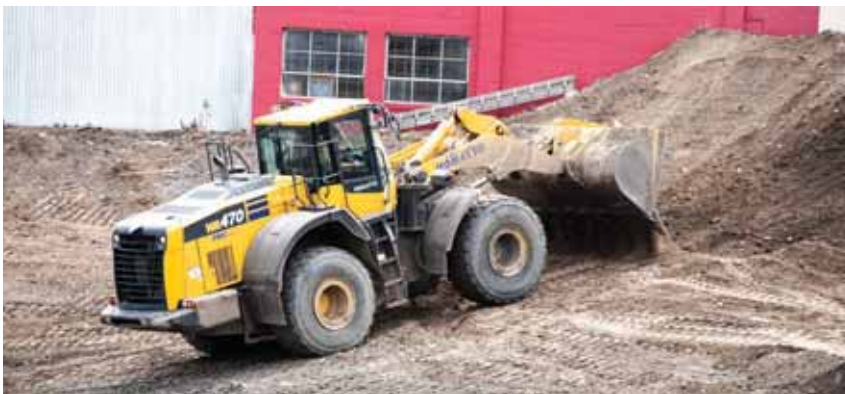
This Zak Dirt operator places material and smooths a bank with a Komatsu WA470 wheel loader on rent from Power Motive.
